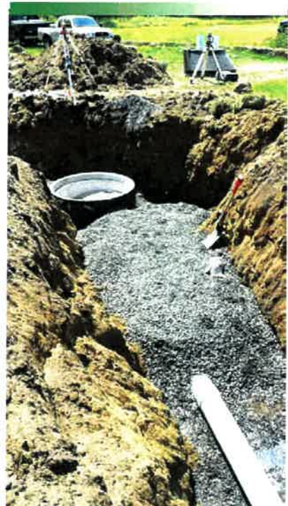
Construction inspection is vital to ensure the project is constructed in accordance with the approved plans and with industry standards.
