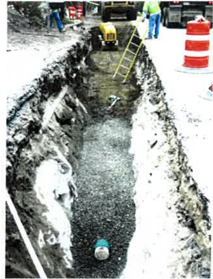
Proper installation and testing will ensure that constructed facilities perform as intended
