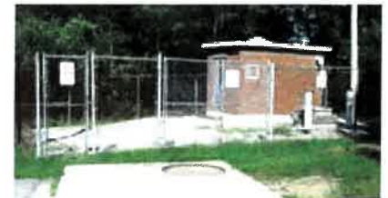
Camp Street Pump Station
